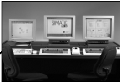
Supervisory Control (SIMATIC PCS: Process Control System)
