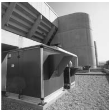
Air conditioning application
